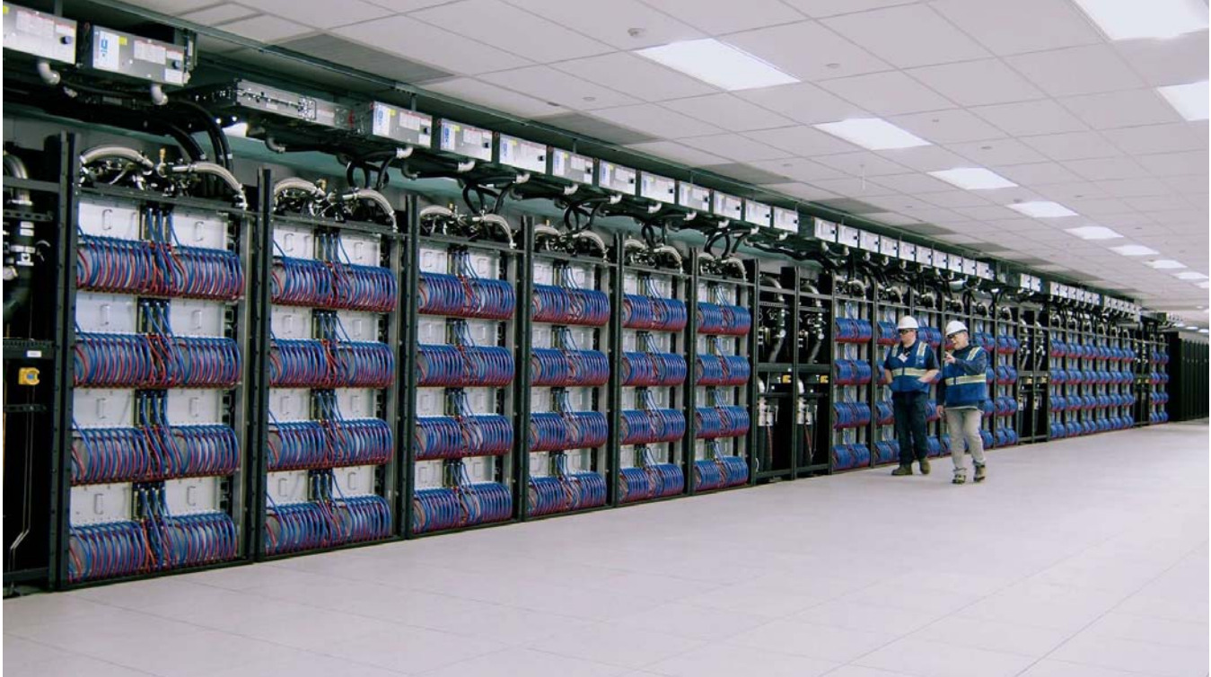
Figure 1: Argonne National Laboratory's newest supercomputer Aurora is currently being installed for operation in 2023/24. Introduction to High-Performance Computing will look at systems like Aurora and answer questions such as what is it made of, how does one program it and how is different from my laptop?
